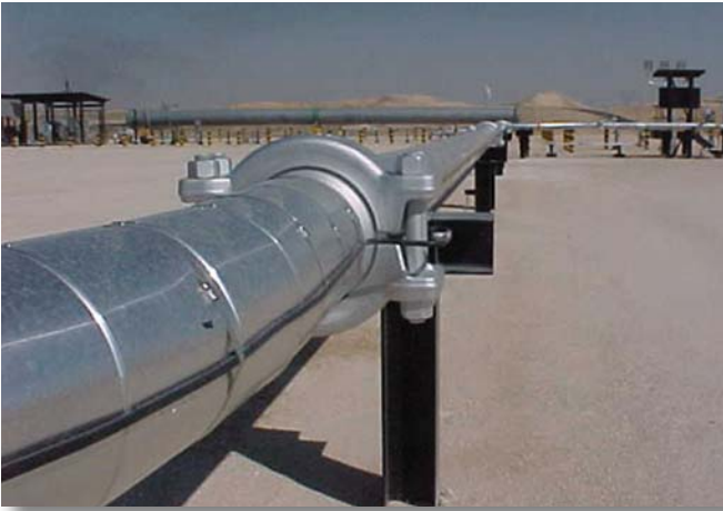
API 10000 psi Flowline
